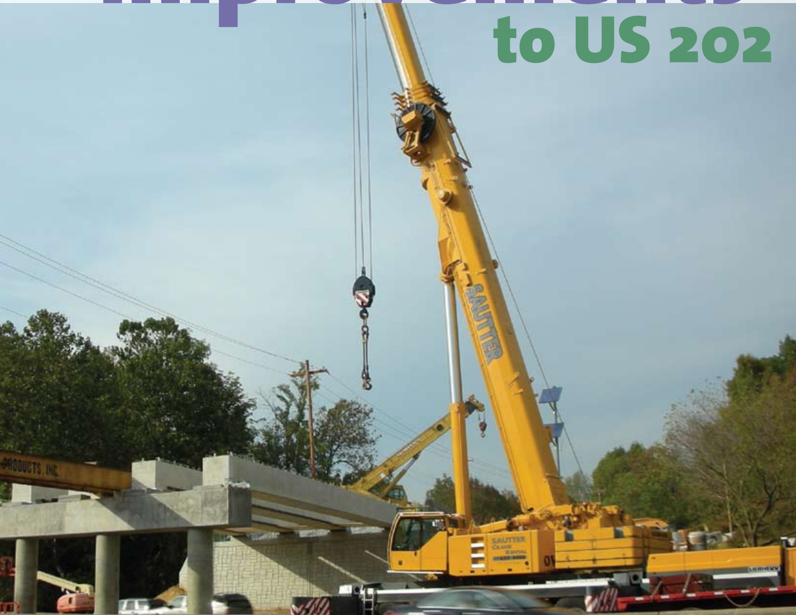
Heavy lifting at the Mill Lane overpass: Beams were set in 2007 for the new bridge over US 202 in East Whiteland Township.
